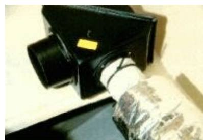
Picture 2: The three way splitter plenum is installed, following the procedure to preconnect insulated flexible ducts. A splitter plenum is a manifold chamber, preferably insulated, with one inlet and several outlets. A distribution plenum is a chamber used to connect a duct to a delivery grill.
