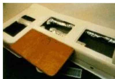
Picture 3: The space under the seat where the air-conditioner and most of the insulated ducts are to be installed. Ducts cannot be strangled or run in sharp bends as air needs to flow freely.
