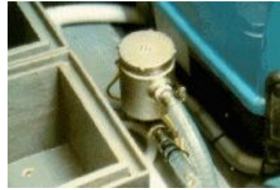
Picture 11: The manual valve is installed directly on the through hull intake; the sea water strainer is installed immediately after.
