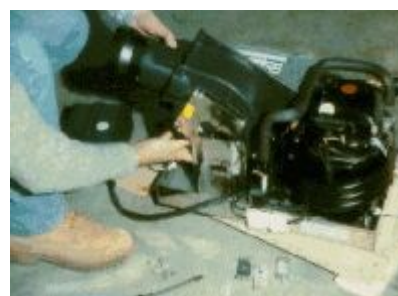
Picture 15: A moment of the installation, when the fan scroll is oriented downwards to fit into the restricted space. A few screws are enough to make the change.
