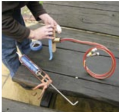
The keel cooler was carefully masked around its outer edges to protect them from excess sealant. Any sealant stuck here will act as an insulator, reducing the unit's efficiency
